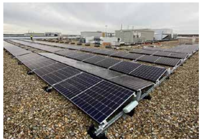
Solar panels at Winnersh Triangle, Reading, UK
